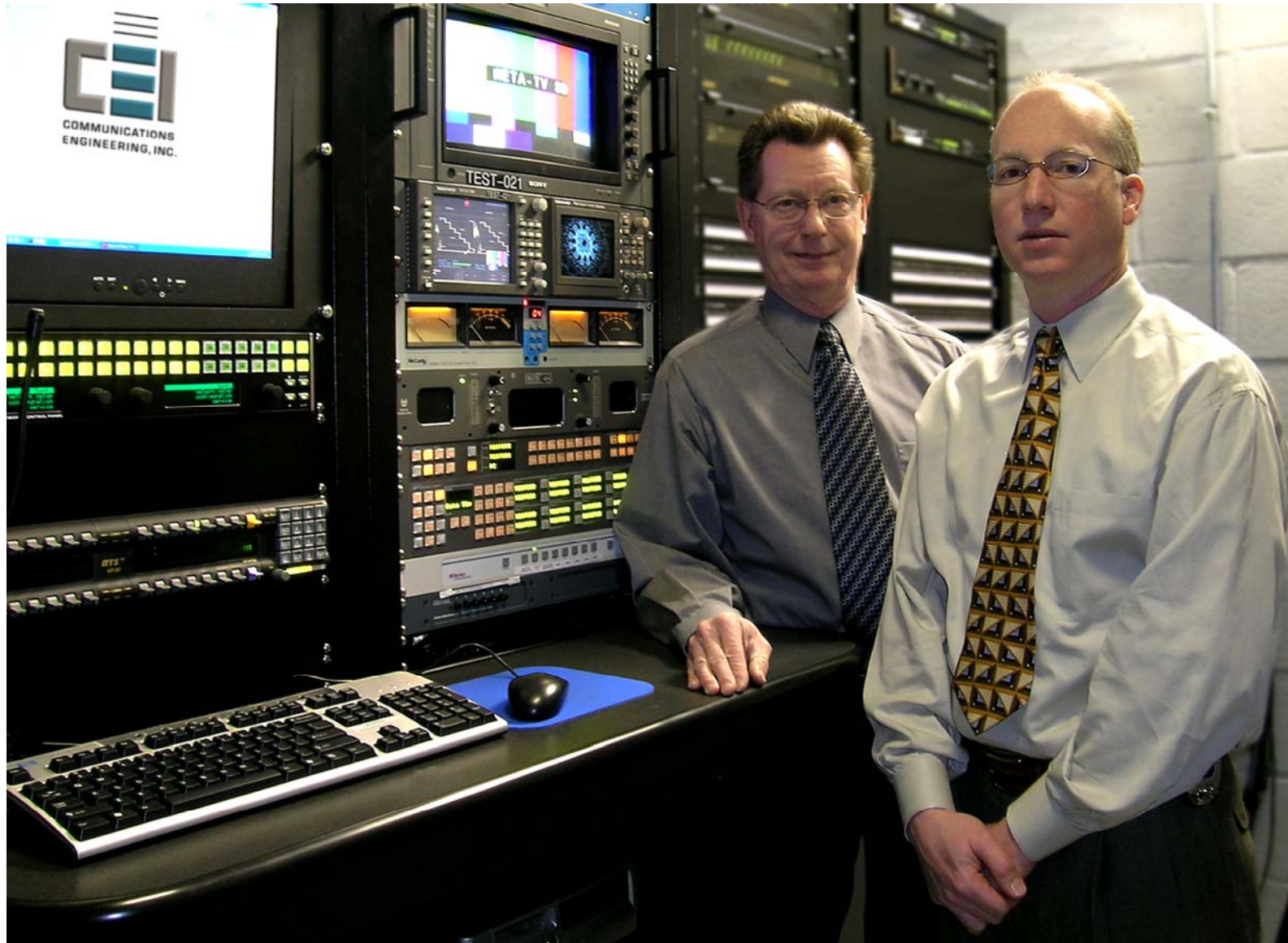
From left to right: Ed Kennedy, WETA's Director of Engineering and Technology and CEI Senior Project Manager, Joe Strobel in WETA's recently constructed CEI Digital Control Room.
